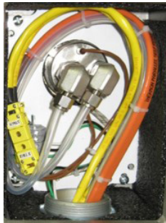
Inside Probe Box
